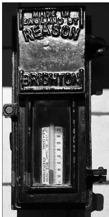
Reason electricity meter
