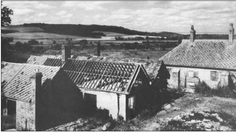
Smithy and loco shed in need of TLC.
