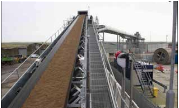
Newhaven aggregate plant
