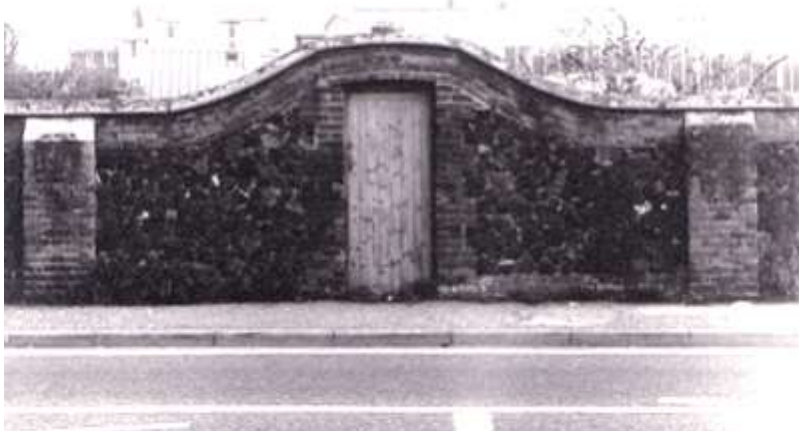
Fig 10. A section of the gasworks wall in Stockbridge Road which includes a doorway. This shews quite clearly the predominant use of retort-linings with brick used for the piers and quoins and lacing courses at the top. The wall is capped with concrete. This section of wall was demolished after 1996 when the site was sold to McCarthy and Stone. (Author)
