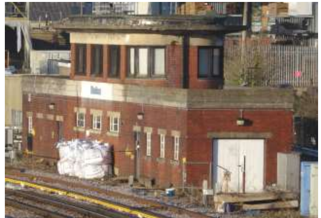
Fig 21. The ‘glasshouse’ signal box at Horsham seen in 2020 when it was in use as a Pway (Permanent Way) lobby. Note the flat roof and projecting concrete canopy. The corner windows in the apsidal ends give all-round visibility. (Author)
