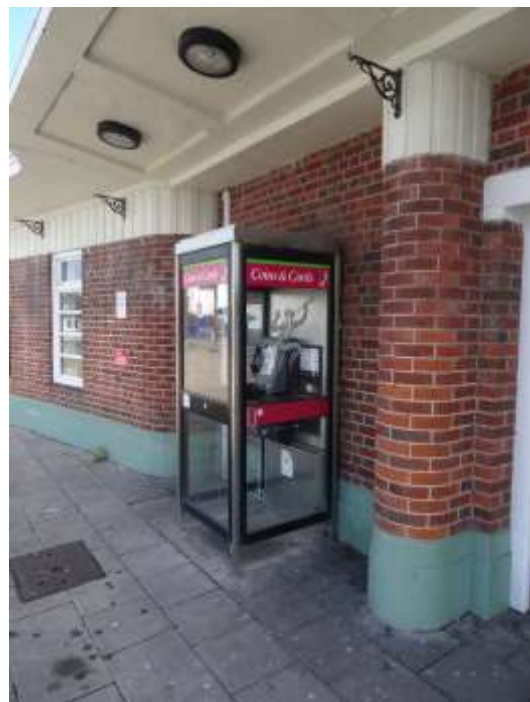
Fig 19. The main entrance is flanked by brick engaged columns, as at Bishopstone, with ribbed capitals – a motif repeated in the frieze of the north wing. All very stylish – apart that is from the rather twee bracket for a hanging basket which is a later addition. (Author)
