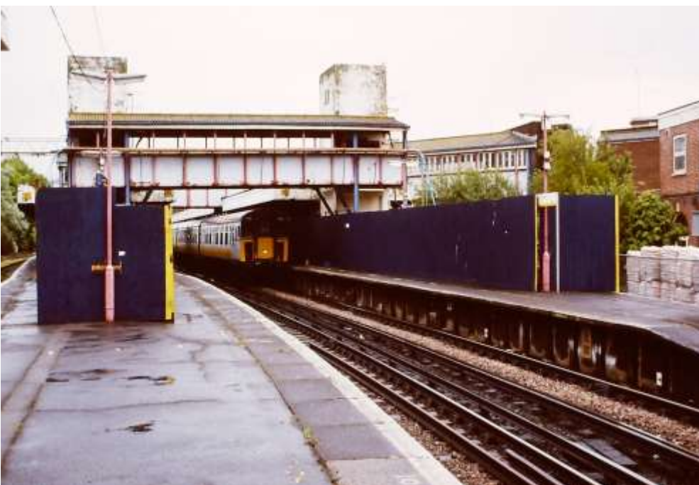
Fig 7. The hoarding along the up island at Hastings bears witness to the fact that this is 2004, and demolition of the Robb Scott buildings is underway. Here we see the neglected luggage bridge with its lift towers, which was about to be swept away, and behind it can be seen the span of the footbridge that linked into the main building, also doomed. A Connex-liveried 4CIG awaits departure for either Victoria or Brighton; no head code is displayed so the driver seemingly has not yet made up his mind. (John Blackwell)
