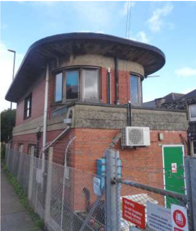
Fig 22. The south end of Bognor box, seen from the road, shewing the rendered platband and the overhanging roof. Severe spalling to the soffit of the latter can be seen – the drawback of reinforced concrete in a marine environment. It is seen in 2020 when it was not only still in use as a signal box but was one of the last outposts of semaphore signalling on the Southern. (Author)
