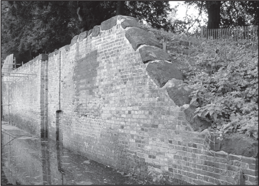
September 2010 showing the east wall of the chamber with scaffolding removed and most of brickwork and coping stones repaired or replaced
