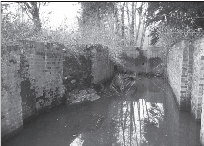
30th August 2006. As the lock looked prior to any work on the chamber walls. Some clearance had begun on the surrounding scrub and trees. The chamber is waterlogged.
