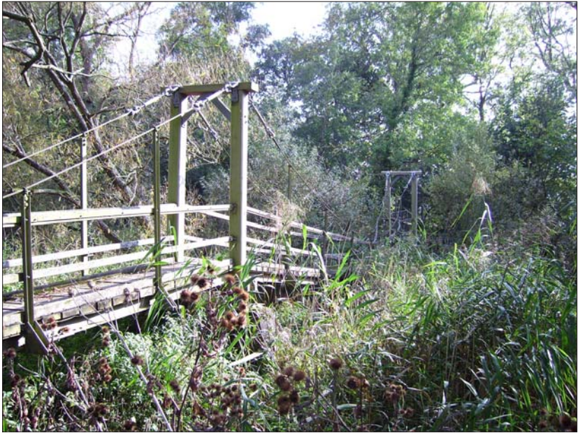
The collapsed suspension bridge at North Stoke ( A. Green )
