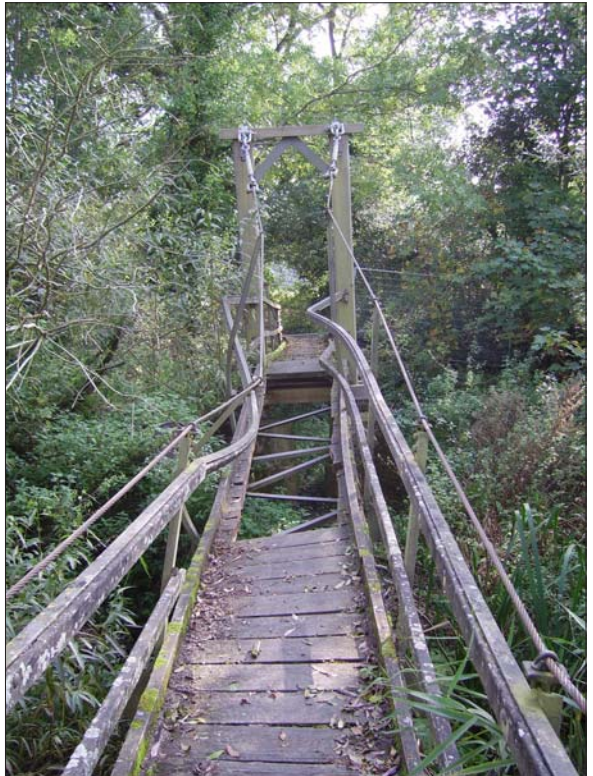
A view across the bridge looking towards South Stoke shewing the damage to the centre span ( Chris Bryan )
