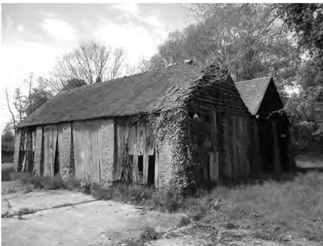
Fig. 6a Warehouse in a state of collapse, 2012.
