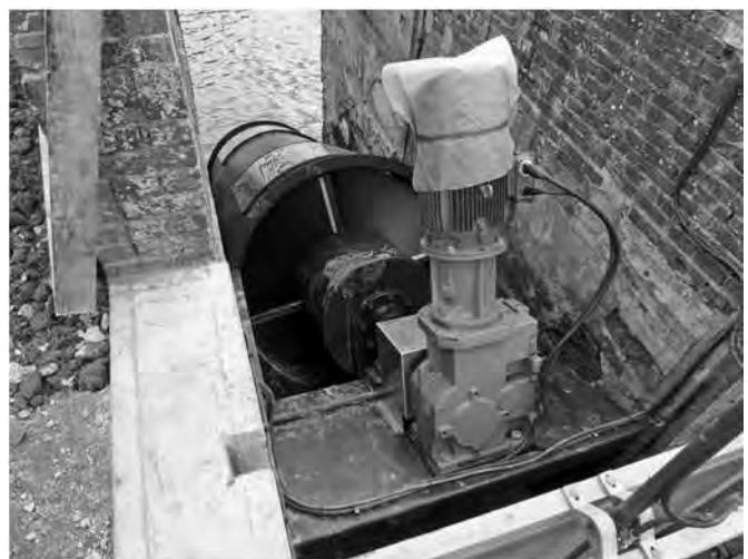
Fig. 5 Turbine in former wheel pit. Archimedes screw driving 15kW generator.
