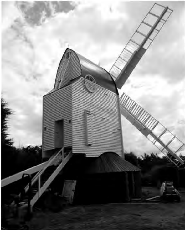
Fig. 1 Argos Hill Mill, external restoration virtually complete, August 2016 (Photo by Philip Hicks)
