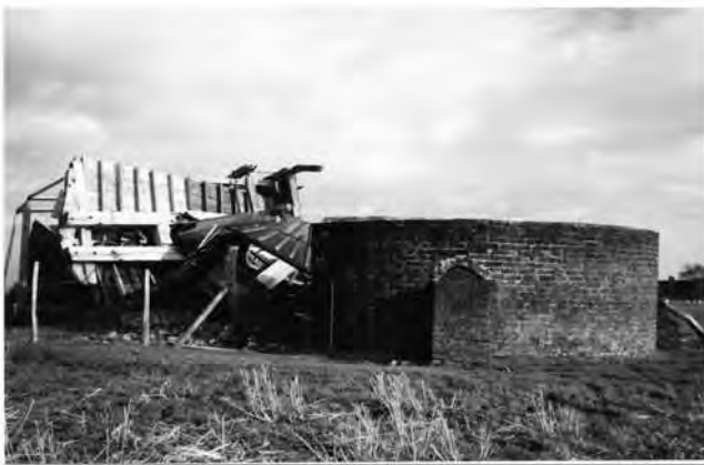
Fig. 15 Winchelsea Mill, collapsed during the Great Storm of October 1987 (Photo by Simon Potter)
