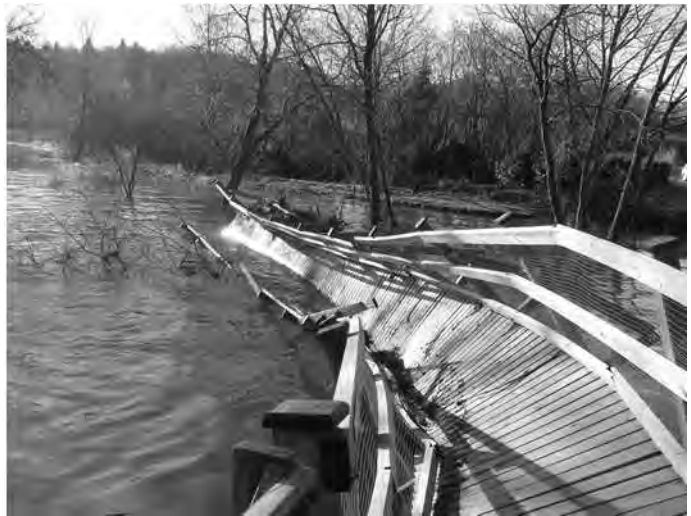
Fig. 7 First boardwalk washed away in the floods of December 2013
