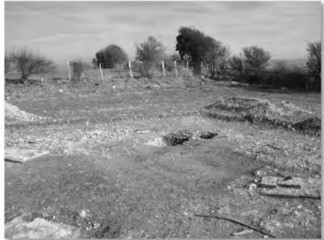
Fig. 13 Ashcombe Mill, the excavated pier foundations of the original mill ( Photo by James Tasker )
