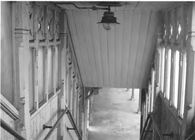
Fig 17. Inside the footbridge at Heathfield – no expense was spared on the elaborate timber mouldings. The peeling paint illustrates the principal drawback with Myres' designs; the high cost of maintenance. (Author's collection)
