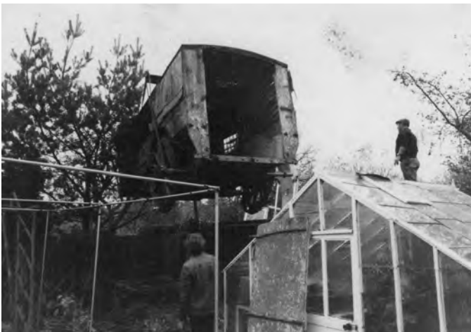
Fig. 6 Steady as she goes! Coppard's team lift the van gingerly over the wall.
