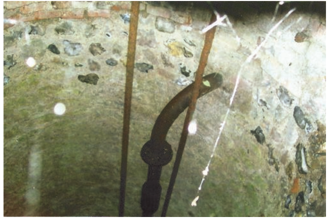
Fig. 14 Pipe running up the inside of the well
