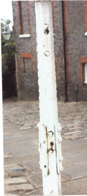
Fig. 8 Crude repair to post (author)
